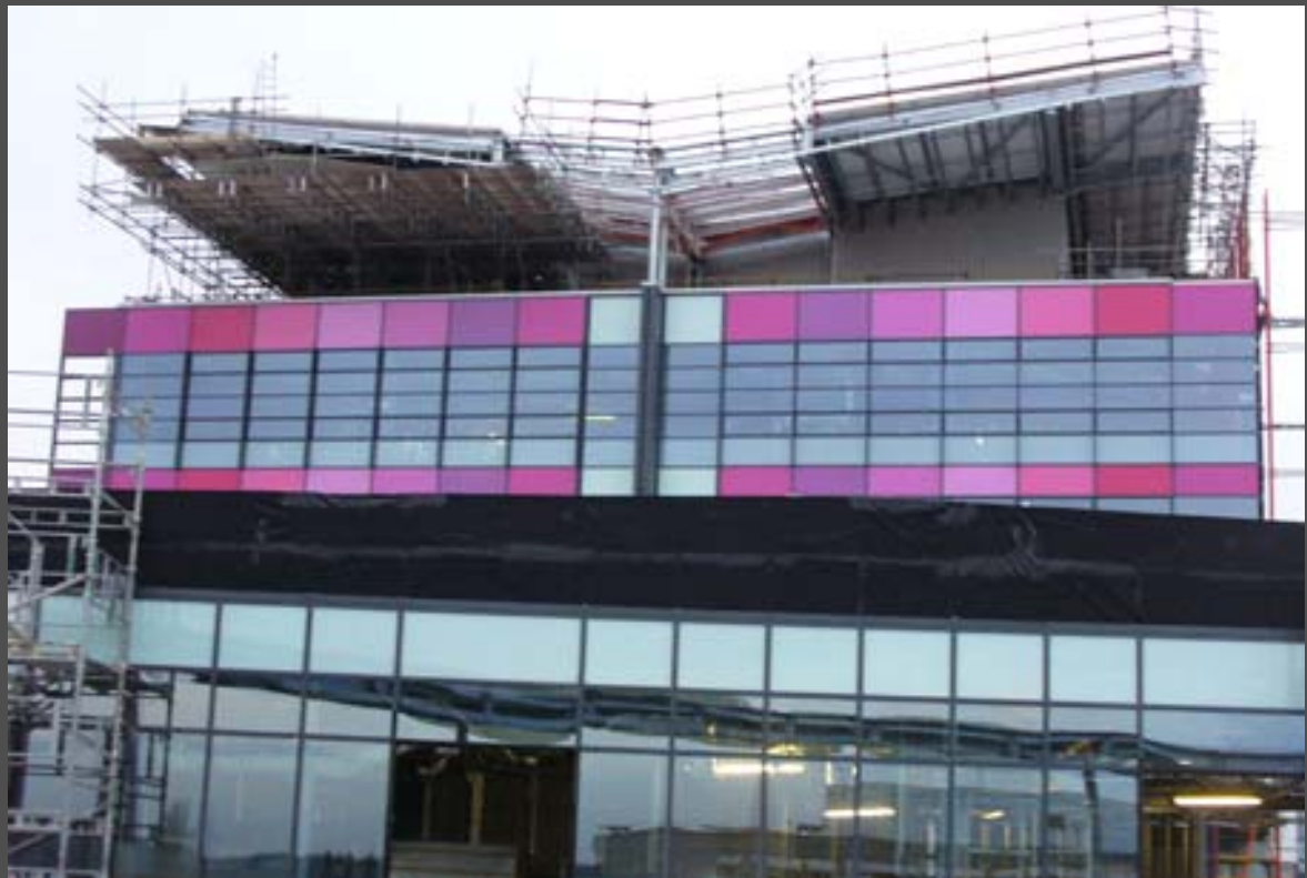
View from the Children's play area to the third ward block tower where the roof is nearing completion
